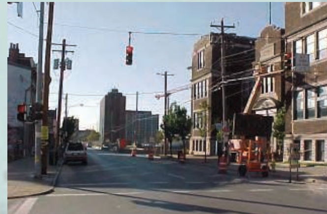
Construction of the first phase of the Calhoun Street Redevelopment began this fall.
